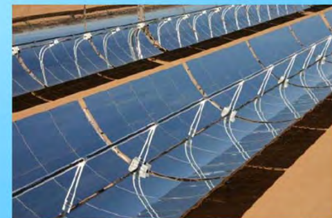
Schott Receivers at APS 1-MWe Trough Plant
